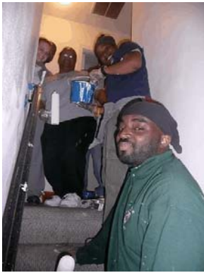
Ignacios Villas Fairfax Youth Probation Officers paint the interior of Midship, a townhome in Burke, VA.
